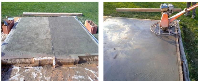
Fig. 2. Mix extended in the slab (Left); Mechanical scrubbing with concrete helicopter (Right).
