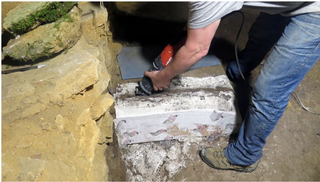
Fig. 8 Photo showing use of a reciprocating saw with a diamond blade to cut the 2 cm-wide kerf separating the block from the rest of the bench
