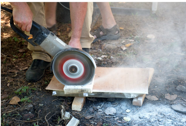
Fig. 16 Using an angle grinder with a diamond blade to cut blocks into columns
