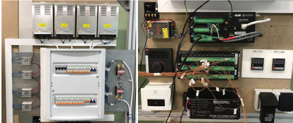
Figure 5. Electrical protection, DC power supply and SSRs (left) and PID controller and datalogger (right).
