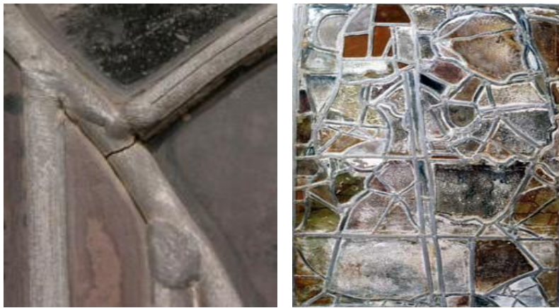
Figure 1.5: (Left) Fatigue crack in lead came. ©Geoffrey Wallace Stained-glass. ©stainedglassausitn.com. (Right) Crusts formation on stained-glass window. Cartuja de Miraflores Burgos. ©Maria Angeles Villegas.
