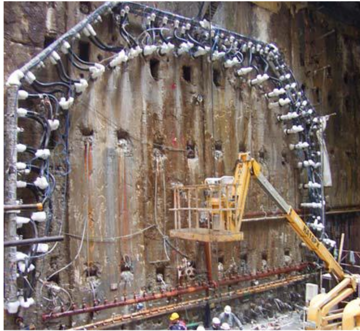
Figure 2.1: Freeze pipes around a platform tunnel in Naples (Viggiani and De Sanctis, 2009)
