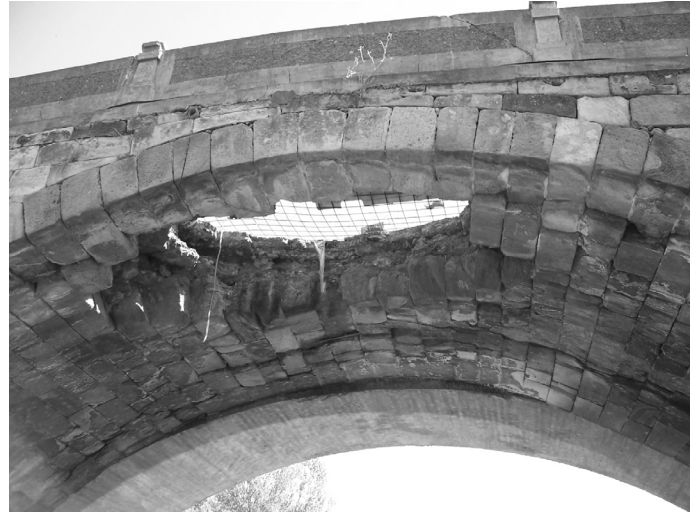
Figure 13. Collapse of the key section of the arch.
