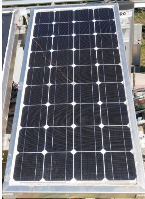
Figure S.26: Third PV/T prototype installed.
