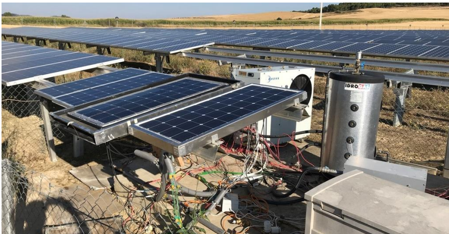
Figure S.31: Final design of the hybrid solar panel test installation.
